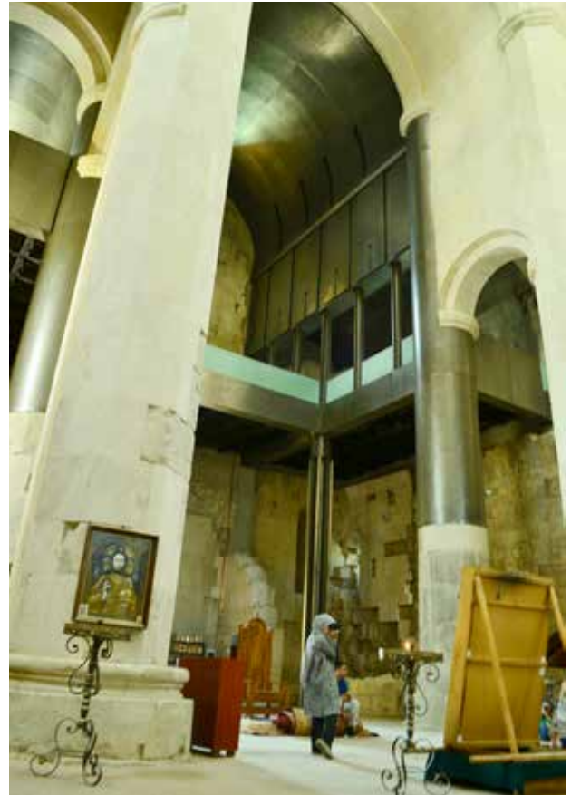
Fig.4. During the contemporary period, the dramatic Frames had been added, in the height of human vision, to the old monastery building in Bagrati's Cathedral in Kutaisi. Georgia. Photo: Zohre Shirazi, Archive of NAZAR research center, 2013.
