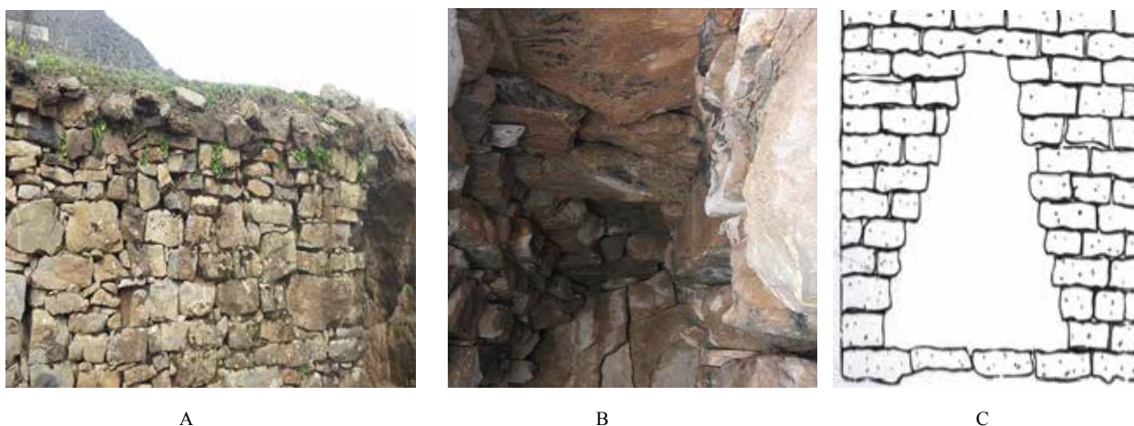
Fig. 3. A, B: Exterior and interior facade of rocky basement in Nowdesheh. Source: author's Archive. C: comparison with complementary schematic design of "arch" from rock. Source: Zomarshidi, 2008, 19.
